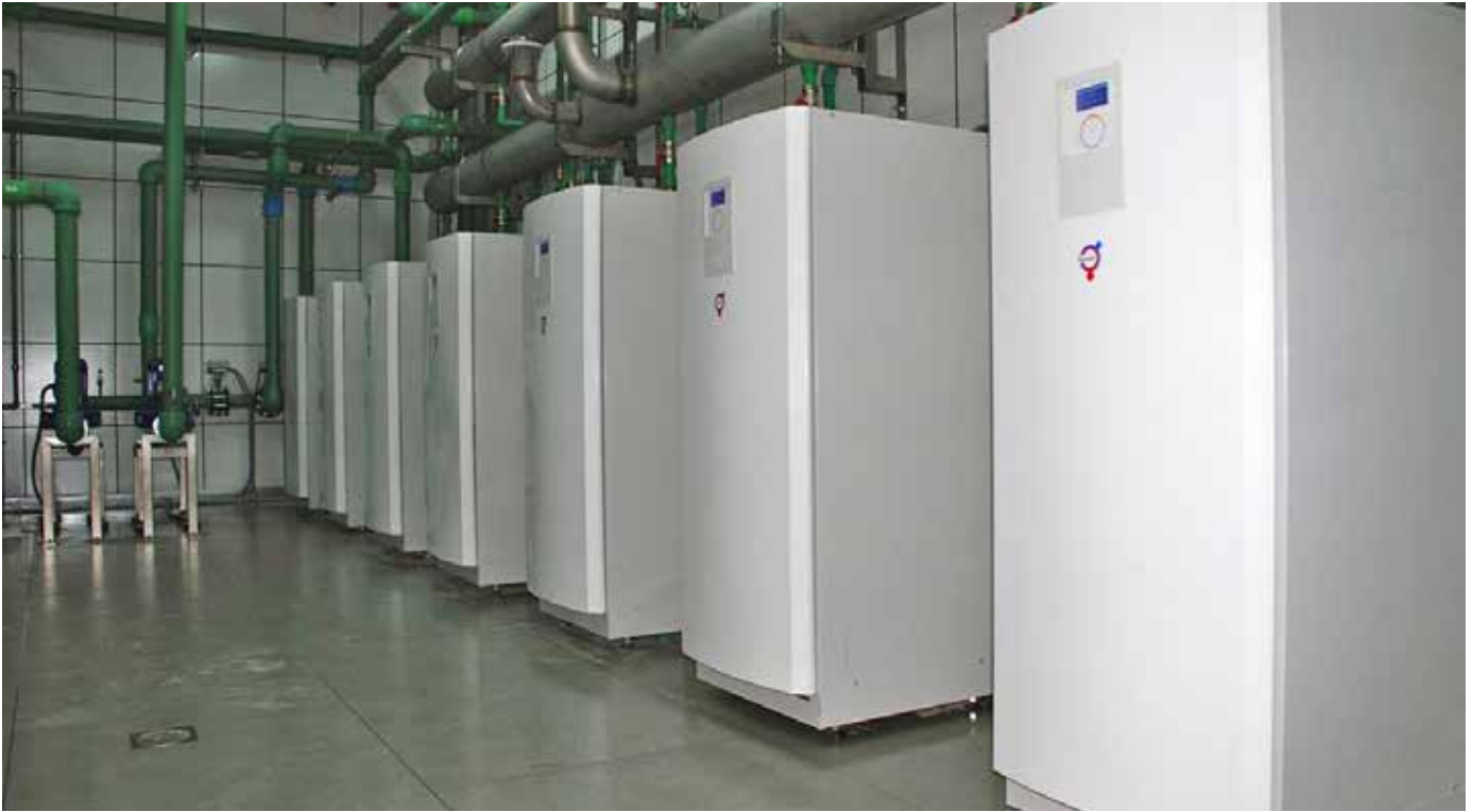
The heating room with Thermia Robust ground source heat pumps
